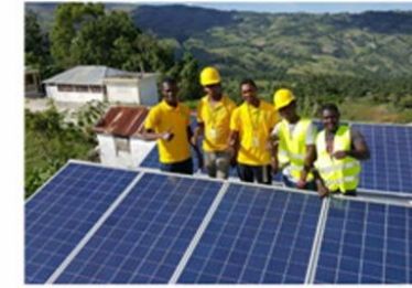
Port-Au-Prince Haiti 3KW
